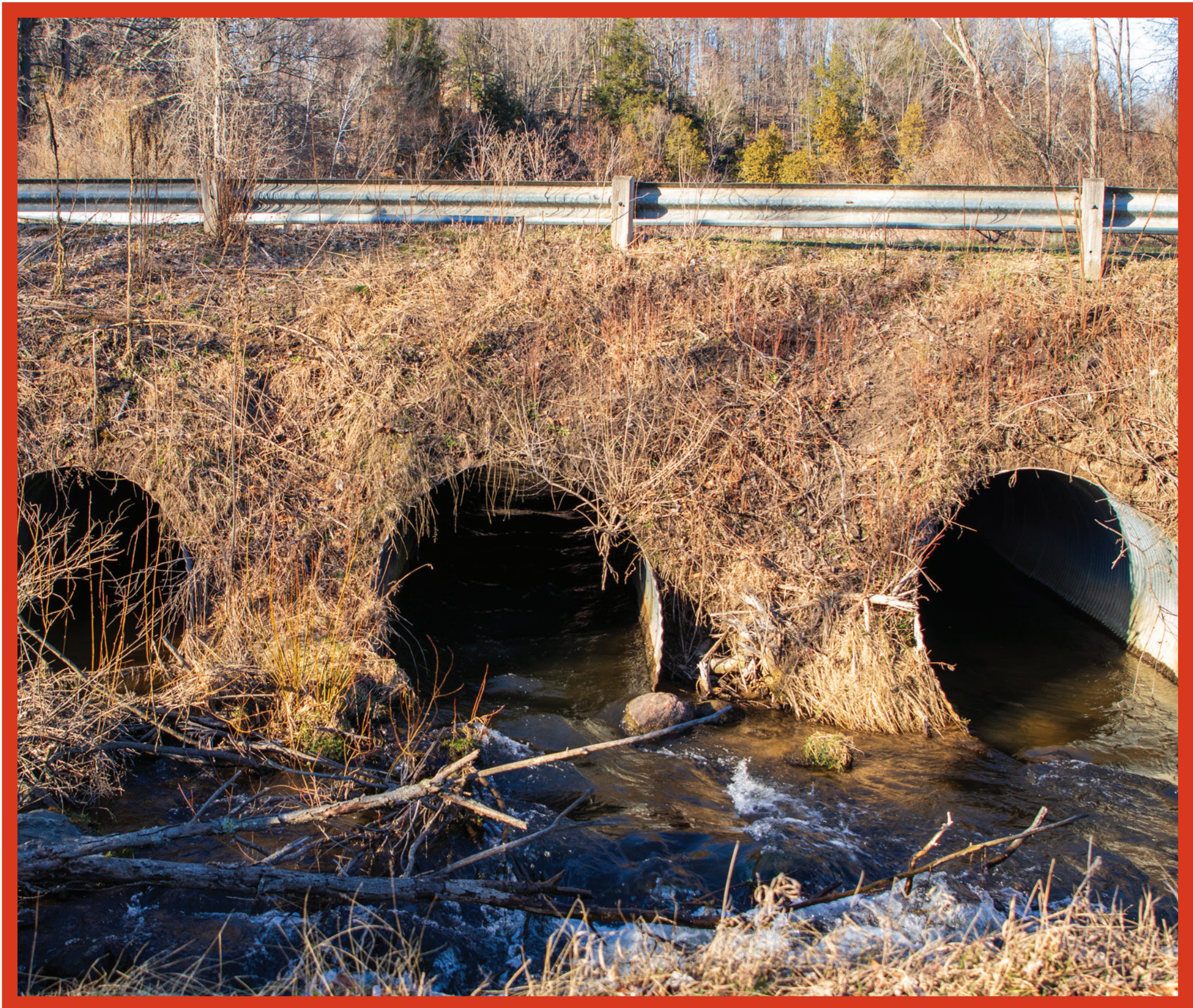
Before: Undersized culverts under Marshville Dam County Road restrict the flow of Stony Creek.
